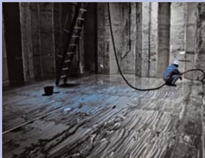
Cleaning job in the stainless steel tank of a JTE tanker. Photo Bruinsma
